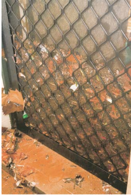
Floodmarks at residence entrance on Victoria St.
