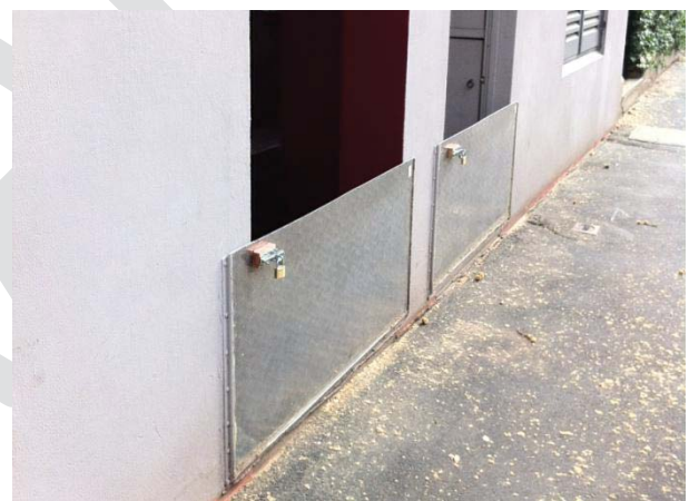
Photo 20: Examples of flood barriers located at commercial premises on Victoria Street.
