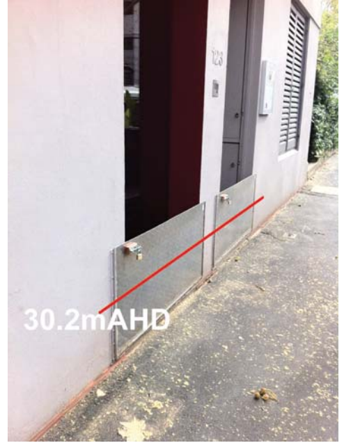
Floodgates installed to avoid inundation at Victoria St, with approximate elevation of flooding in February 2010.
